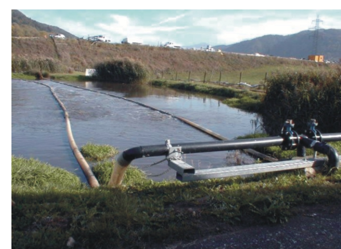
The wastewater plant was built in 1989 as a ventilated pond purification plant.
