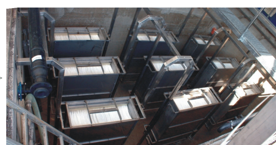
The modules have been situated in an existing basin used as fixed-bed nitrification in the original plant design.
