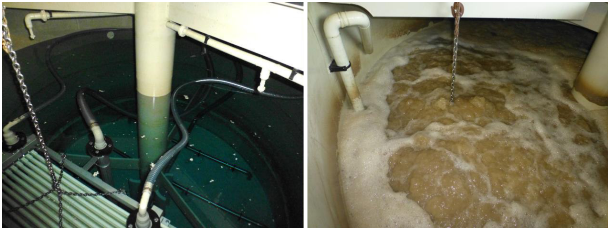
Picture 2: MBR-Industrial plant
